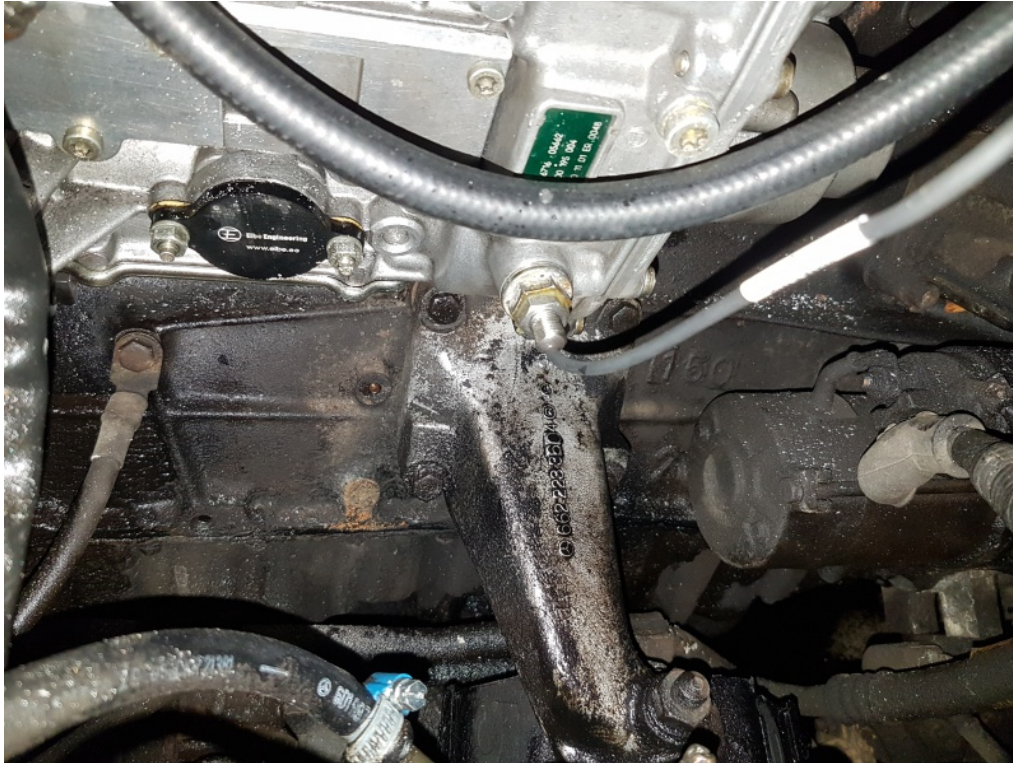
Figure 4.4: Honeywell LCZ260 sensor installed in injection pump
